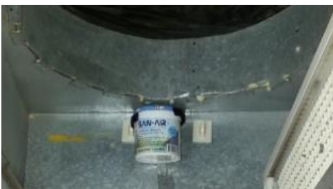
SAN-AIR tm jar installed in return box of ducted air system.
